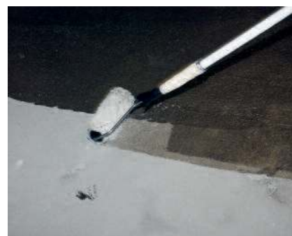
PCI Epoxigrund 390 and/or PCI Epoxigrund Rapid is worked into the prepared substrate e.g. by means of a paint roller.
